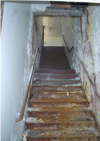
Stair water damage
