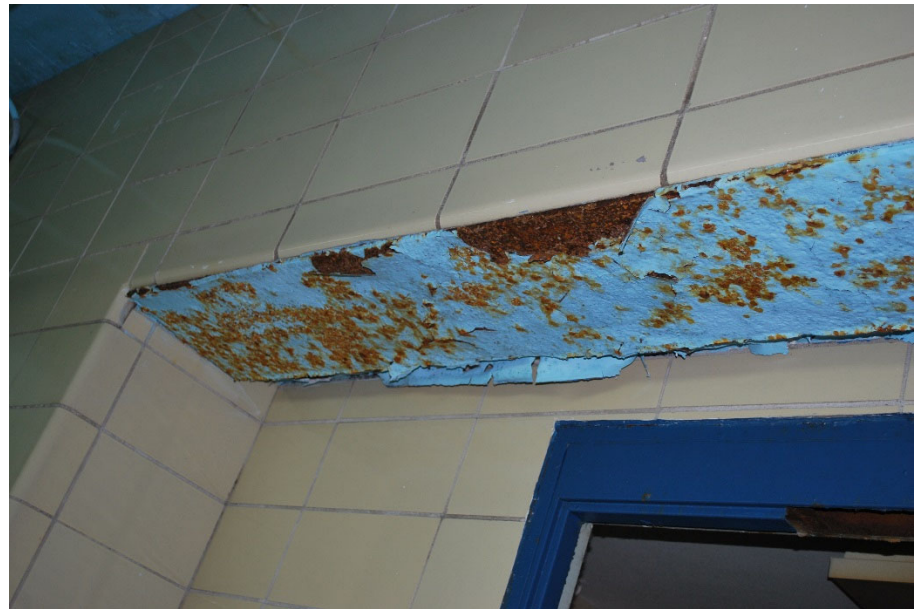
Pool Beam Corrosion
