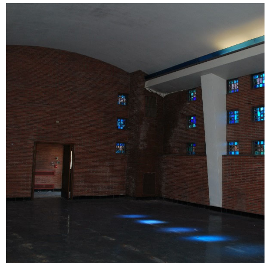
Interior looking at entrance & damage
