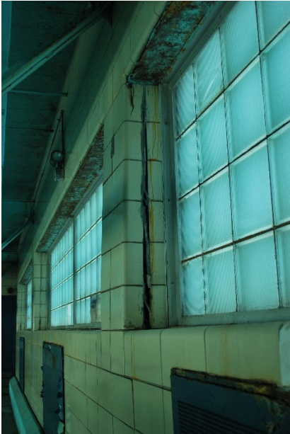
Pool Exterior Wall Damage
